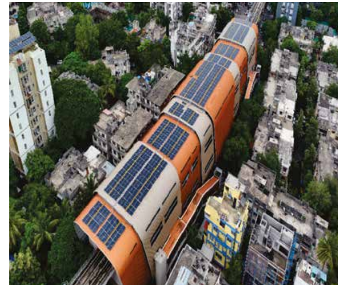
Roof Top Solar Plant
